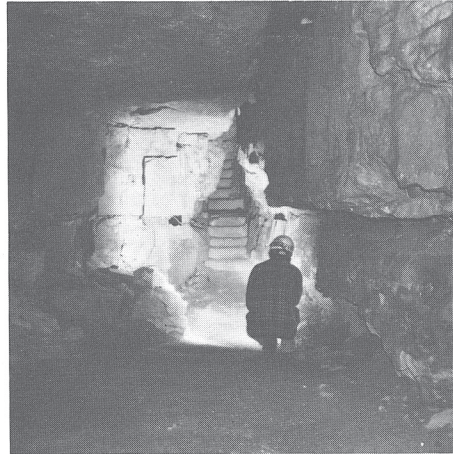
Fig. 5. View of entrance from Reception Room (note enlarged fracture in ceiling).
